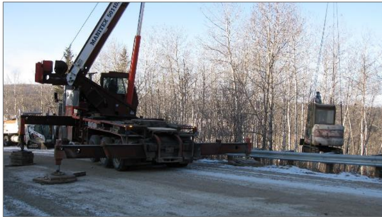
Photo 6 – A mini excavator being lowered onto the excavation area for backfilling activities.
