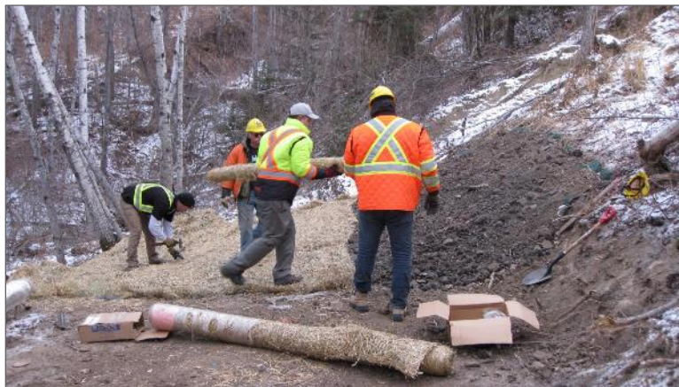
Photo 10 – Installation of the LANDLOK® S2 product over the reinforcement matting to allow for vegetation regrowth.
