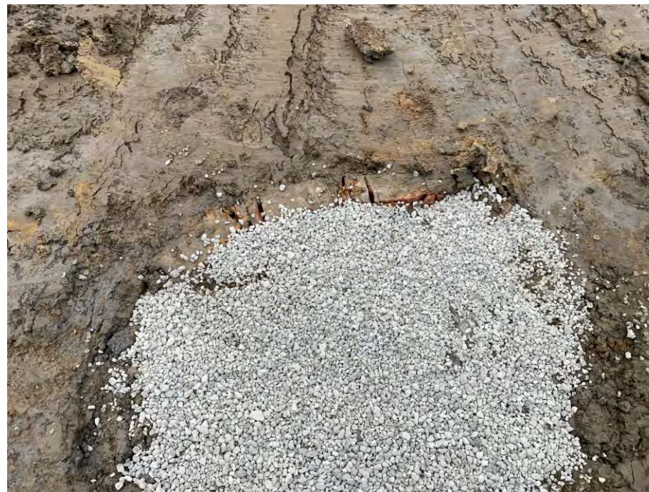
Photo # 3: Exposed decommissioned well (note bricks), sealed with bentonite - November 2021.
