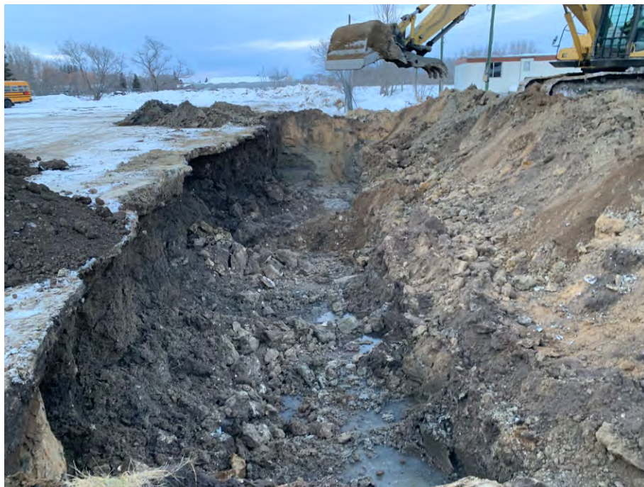
Photo # 5: Advancing excavation into bus garage property, backfill on east side - November 2021.
