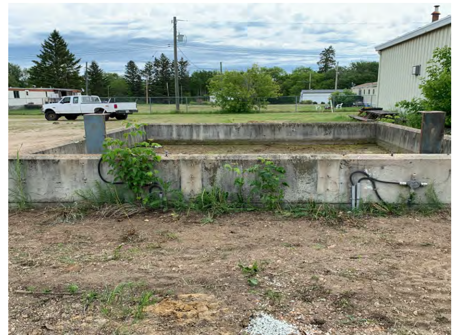
Photo # 3: View of former fuel dispenser location, west side of tank dike (note electrical lines).
