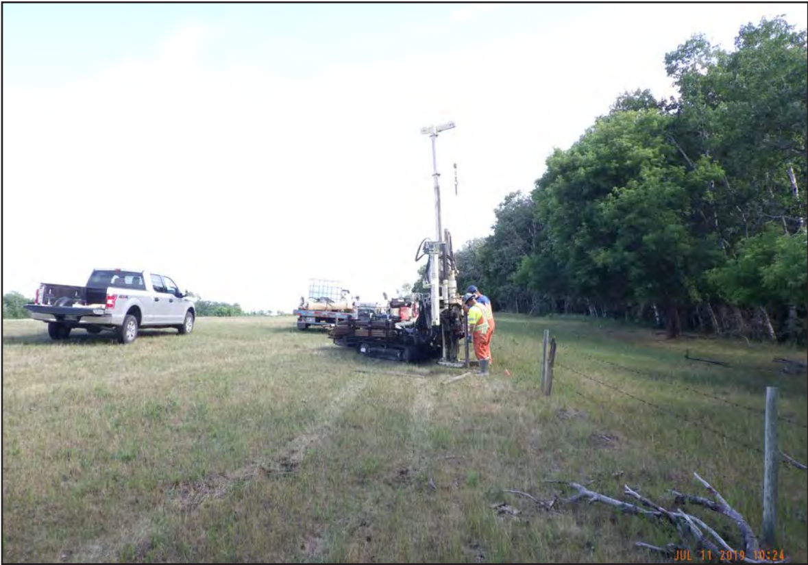
View looking north of monitoring well MW18 being advanced off-site to the north of the IWWTF.
