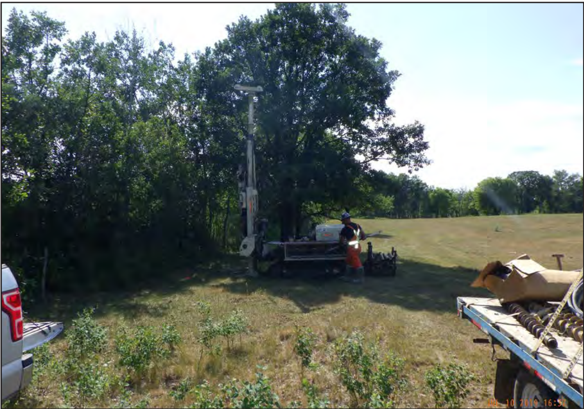
View looking west of monitoring well MW16 being advanced to the northwest of the IWWTF.
