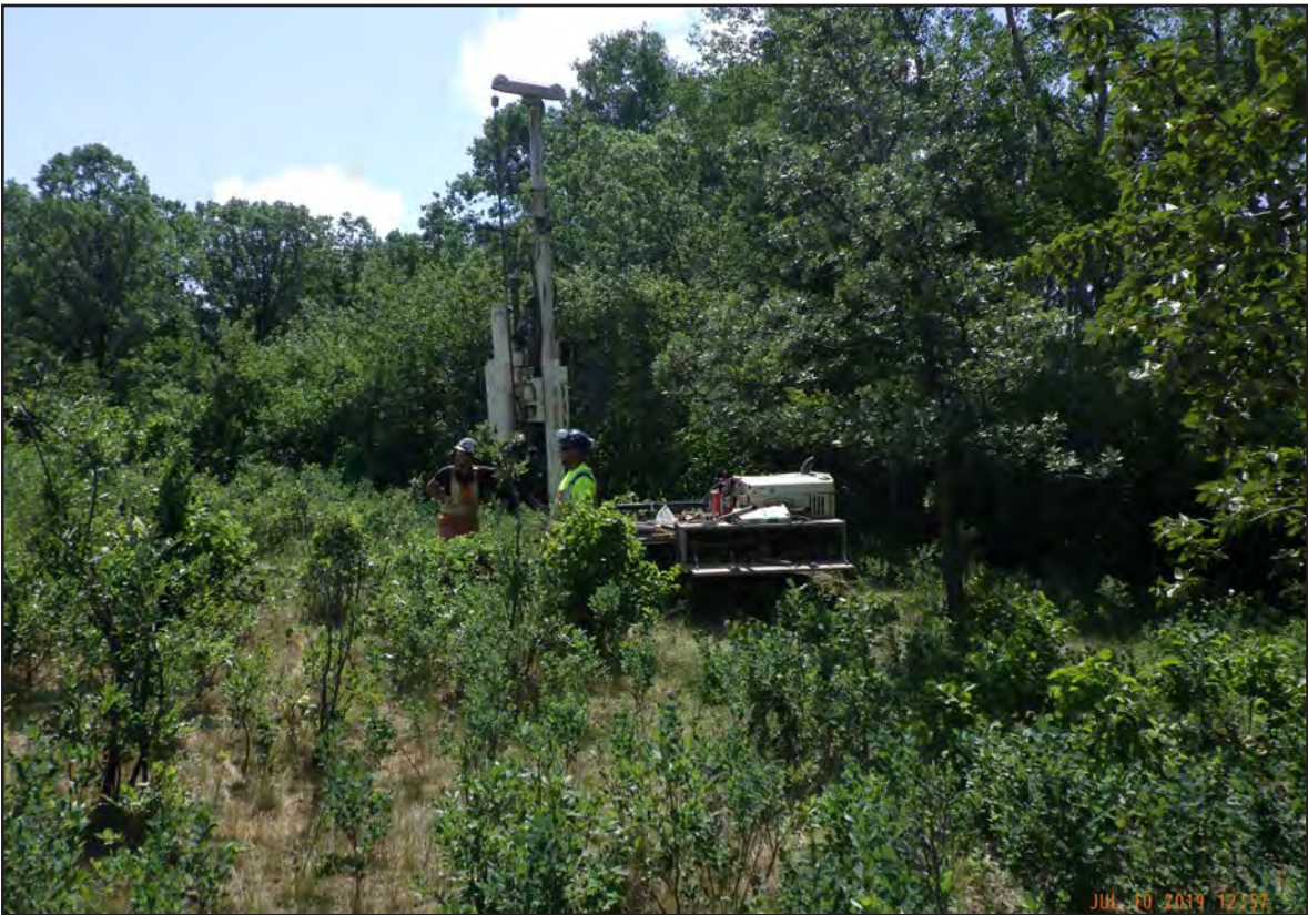
View looking south of monitoring well MW14 being advanced to the northeast of IWWTF.
