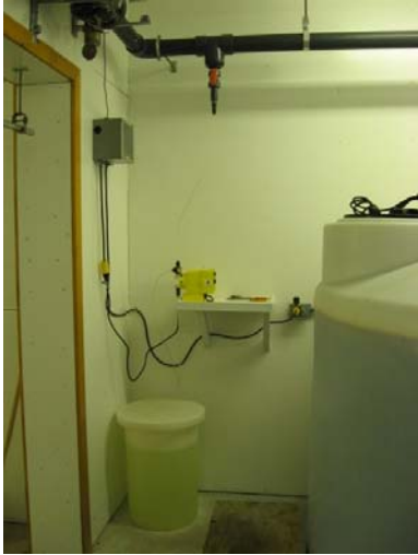
Photo 13. Chlorine injection system.
