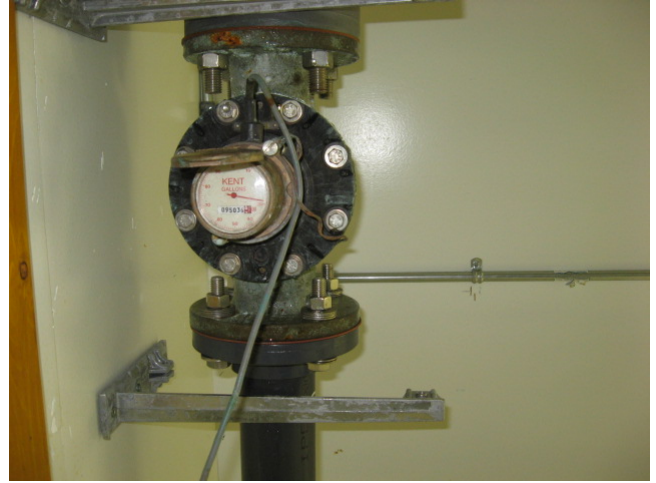
Photo 14. Flow meter monitoring flow into pumphouse.
