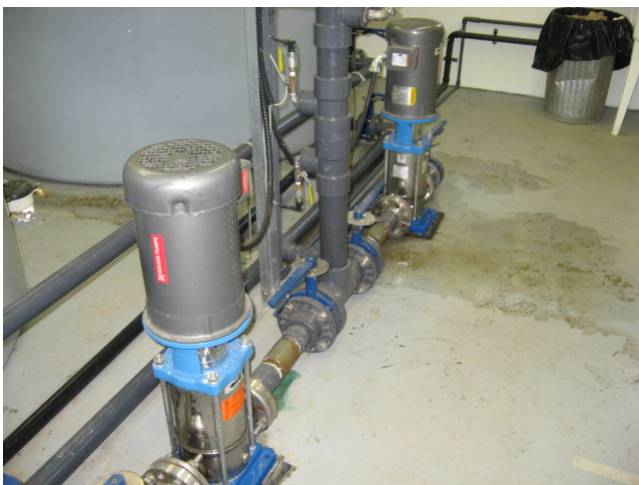
Photo 17. Community supply pumps located within pumphouse.
