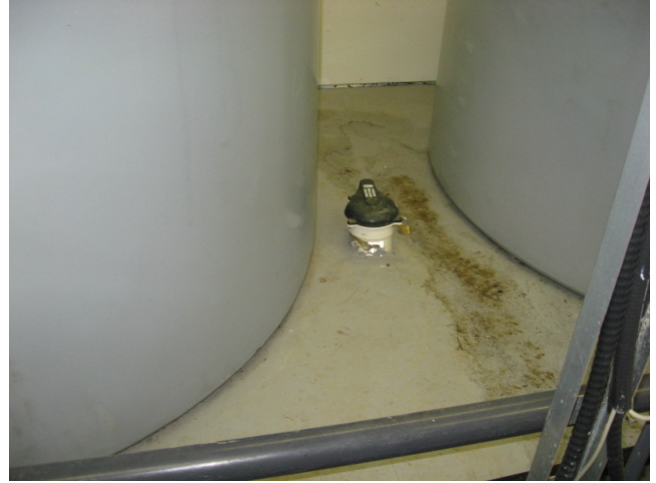
Photo 8. Supply well PW-3 located within pumphouse.
