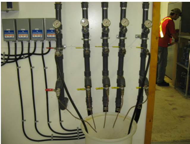
Photo 11. Sampling ports for all supply wells.
