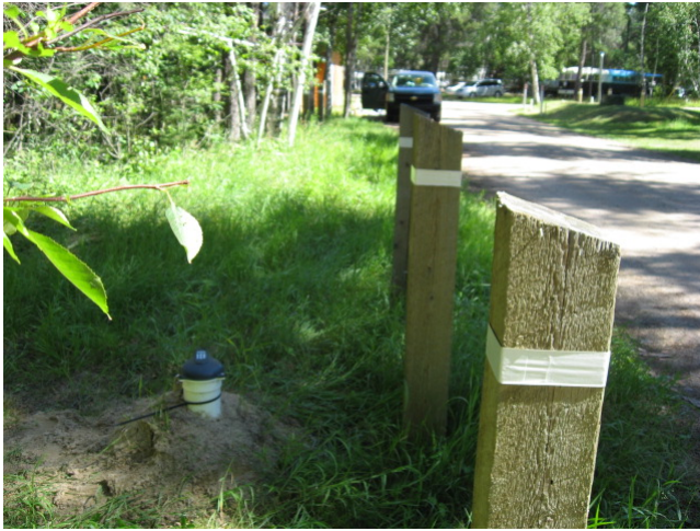
Photo 3. North view of supply well PW-4 and current pumphouse.
