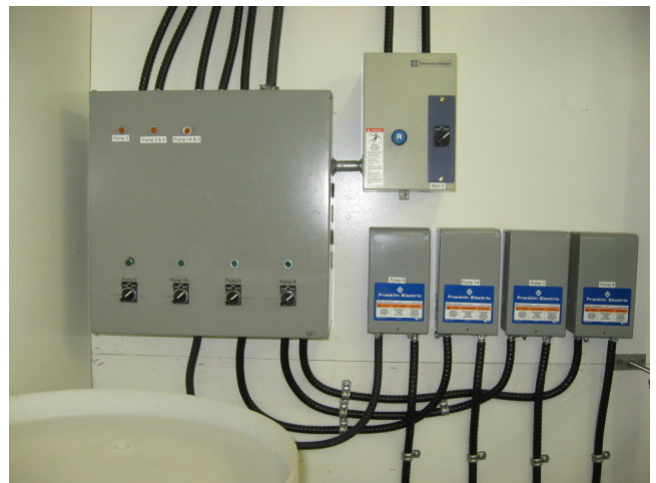
Photo 12. Control panel for all supply wells.
