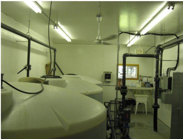
Photo 15. Storage tanks located within the pumphouse.
