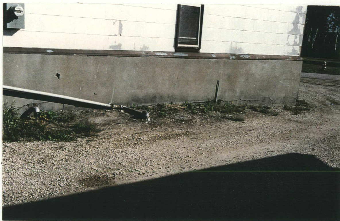
Photo 4 Location of Underground Fuel Storage Tank on the South Side of the Former Diesel Generating Station
