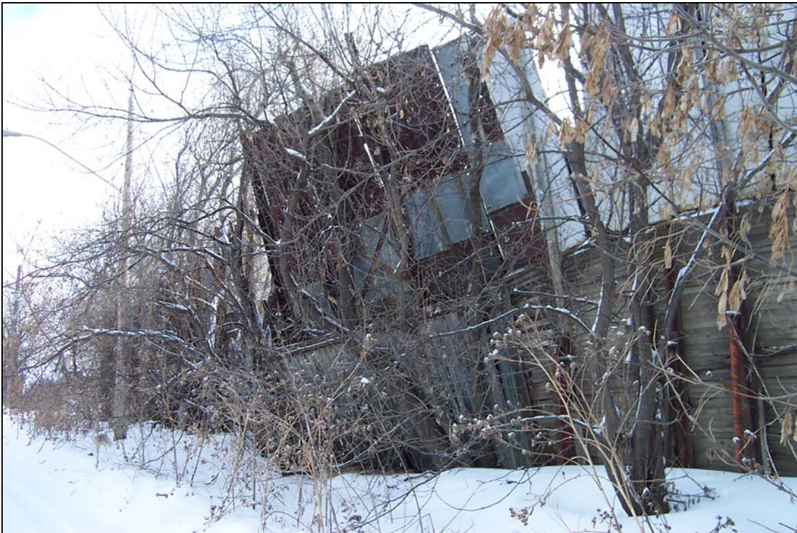
Photograph 6: The fence along the northern property line located at 9 First Street is failing.
