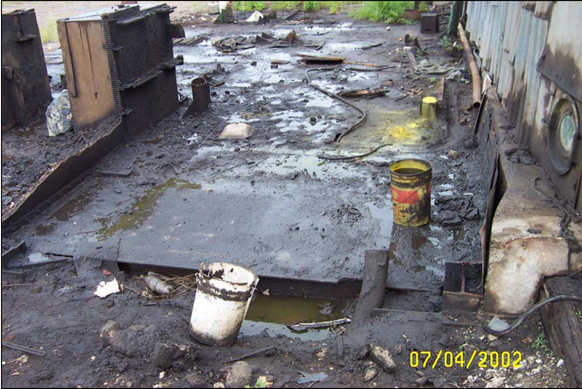
Photograph 21: Area of extensive hydrocarbon staining on and around a concrete pad located within the fenced compound at 9 First Street. Note the yellow 5-gallon pail that is full of what appears to be transmission fluid.
