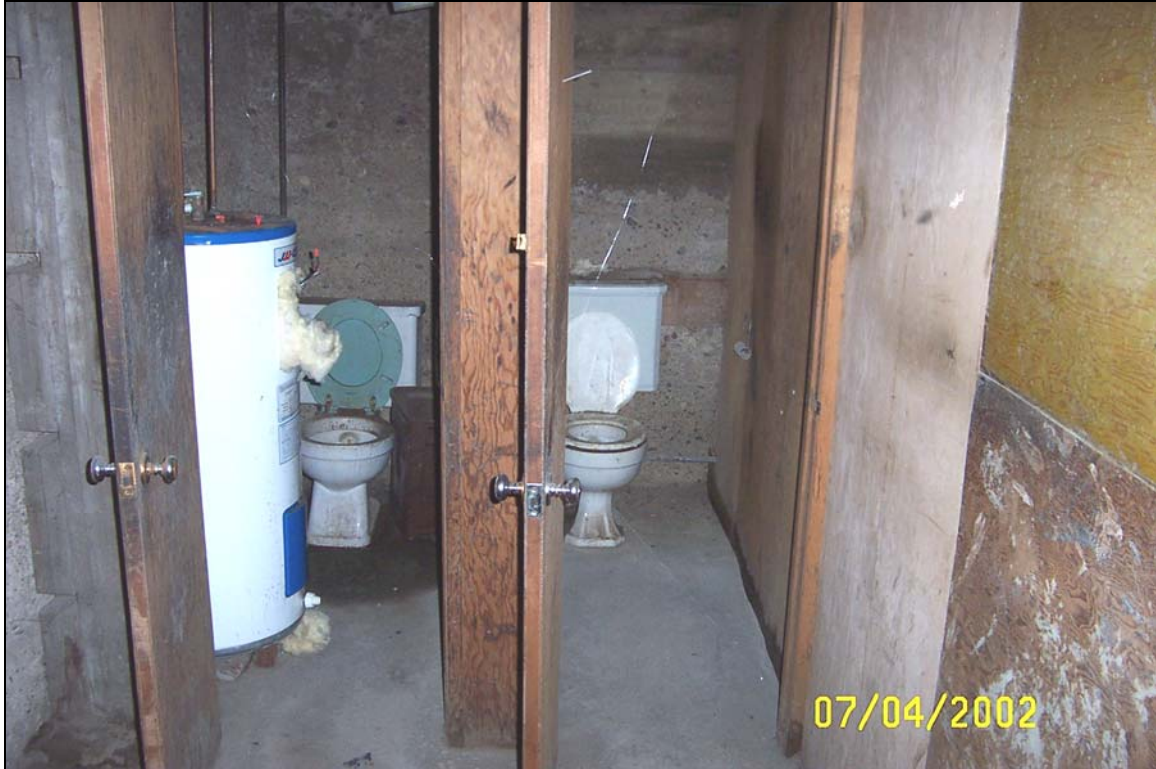
Photograph 13: Washroom facilities are located in the basement east of the furnace room. Note the hot water tank is located in left washroom.
