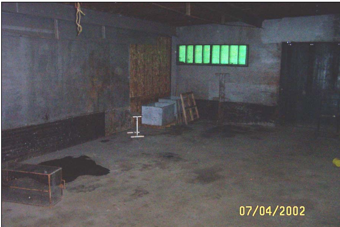
Photograph 14: Looking west into the shipping area. The dark area on the floor to the left of the photograph is a result of water ponding.
