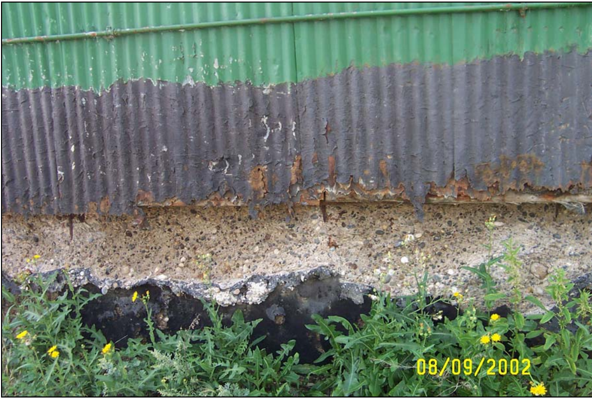
Photograph 17: The exterior of the building along the north wall of the curing area has undergone extensive corrosion, apparent as a result of the salt within the building.
