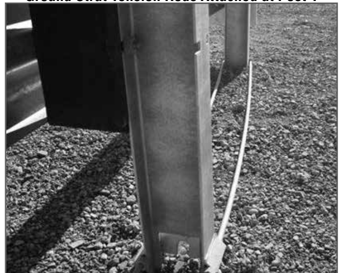
Slight Bend on Ground Strut Tension Rods
