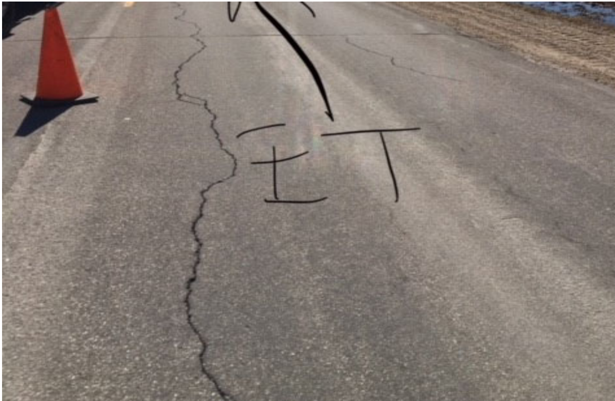
Figure 2.0.5: Top-Down Fatigue Cracking on PTH 67 at PTH 8, Manitoba
