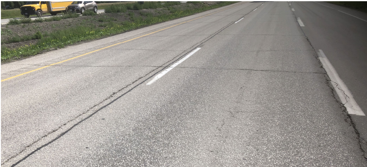
Figure 2.0.7: Reflective Cracking in Composite Pavement on PTH 1 at Whitehorse, Manitoba
