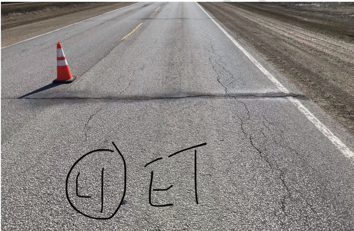
Figure 2.0.4: Bottom- Up Fatigue Cracking in Wheel Path on PTH 2 at Oak Bluff, Manitoba
