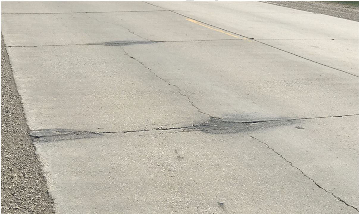
Figure 2.0.10: Longitudinal Cracking in PCC Pavement on PR 207 (North of PTH 15), Manitoba
