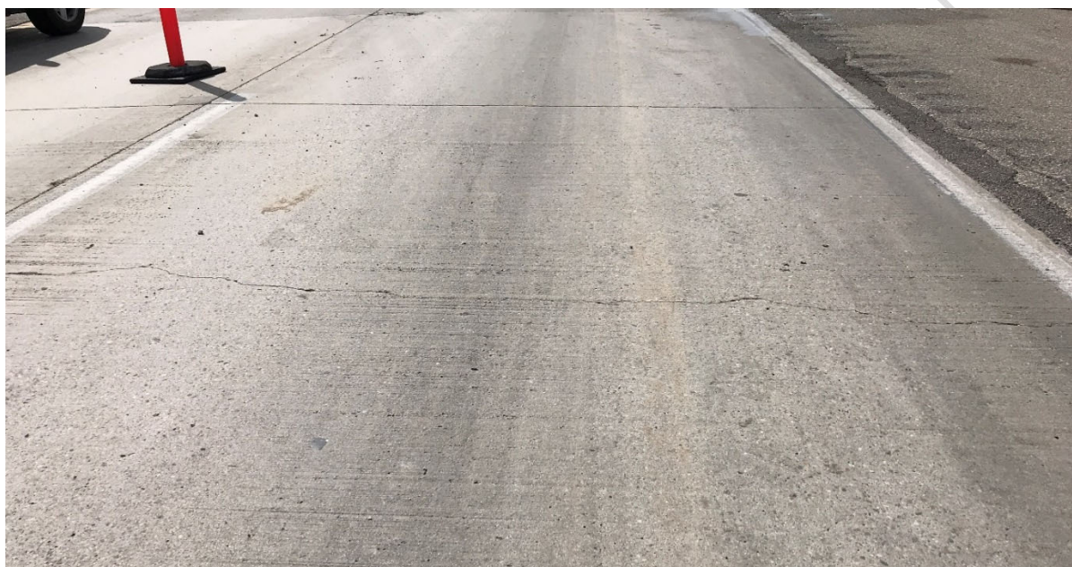
Figure 2.0.9: Transverse Cracking in PCC Pavement on PTH 59S near PTH 100, Manitoba
