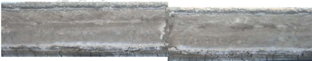
Figure 2.0.8: Faulting in PCC Pavement (produced using Photos from PTH 9, Manitoba)
