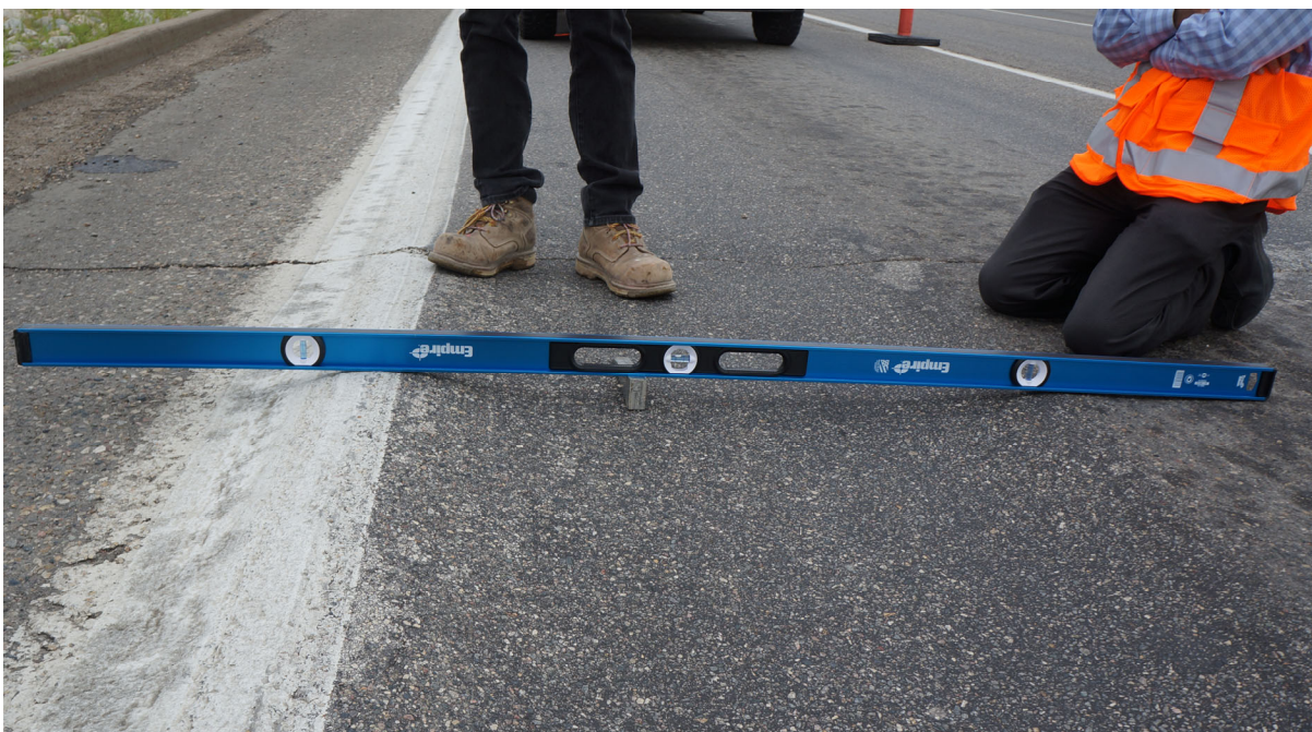
Figure 2.0.3: Surface Rutting on PTH 1 at 1st Street, Brandon, Manitoba
