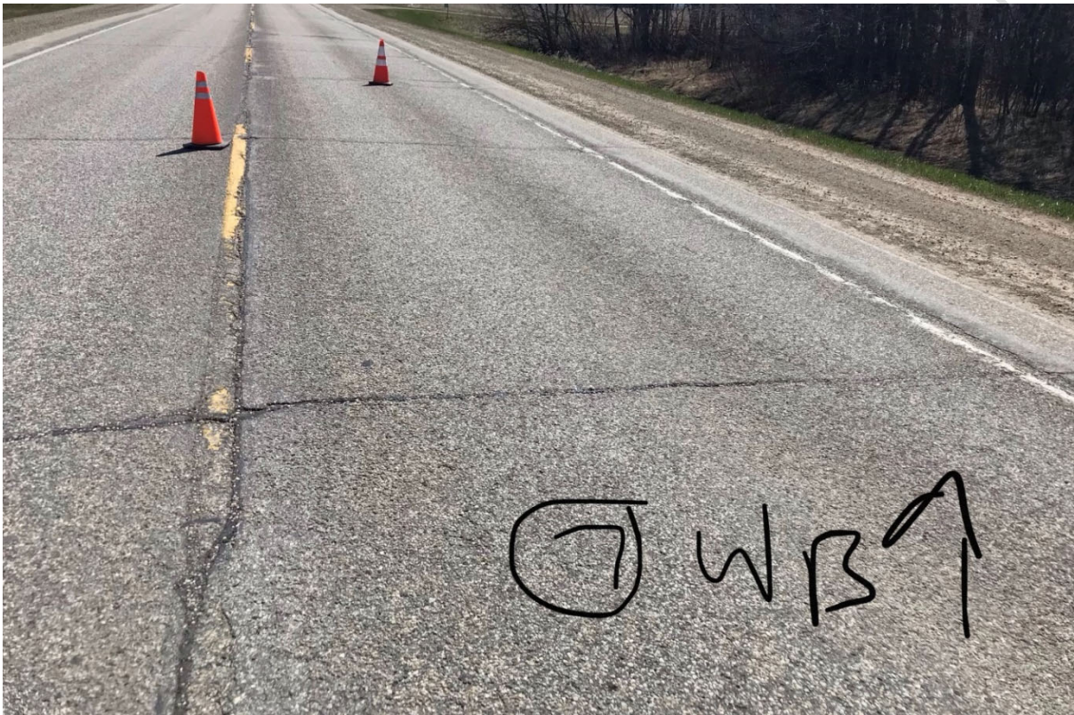
Figure 2.0.6: Transverse Cracking on PTH 23 at Carmen, Manitoba
