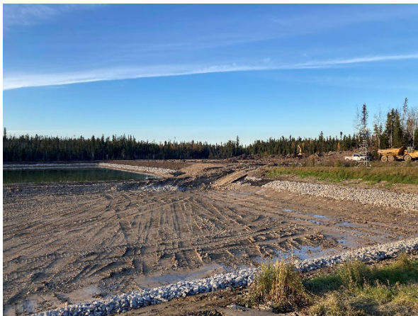
Paint Lake Provincial Park Wastewater Treatment Lagoon
