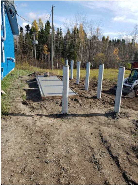
Wabowden Water Treatment Plant Generator
