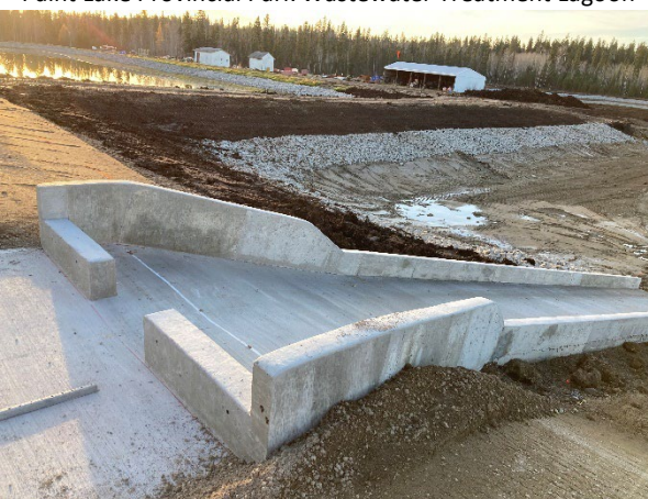
Paint Lake Provincial Park Wastewater Treatment Lagoon
