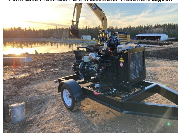
Paint Lake Provincial Park Wastewater Treatment Lagoon
