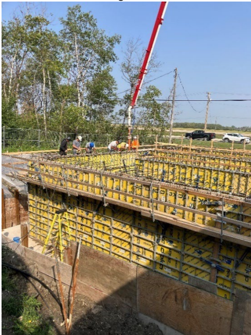
R.M. of Brokenhead WTP Upgrades
