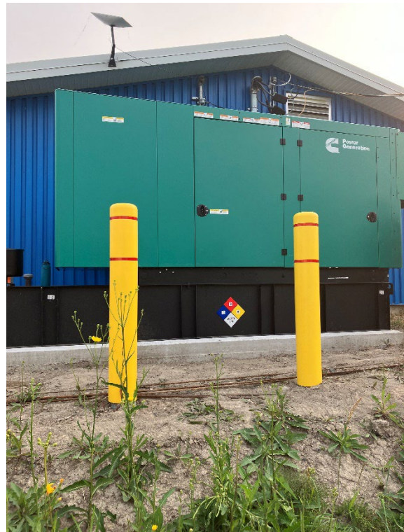
Wabowden Water Treatment Plant Generator
