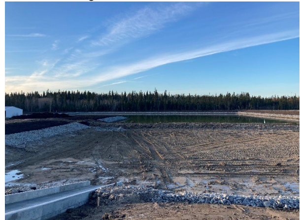
Paint Lake Provincial Park Wastewater Treatment Lagoon
