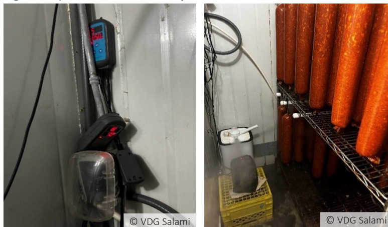
Figure 4 | Humidifier and temperature controllers
